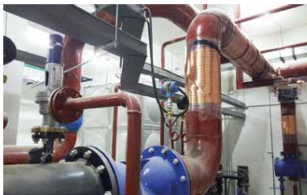
Vulcan S350安装在高区供热系统
