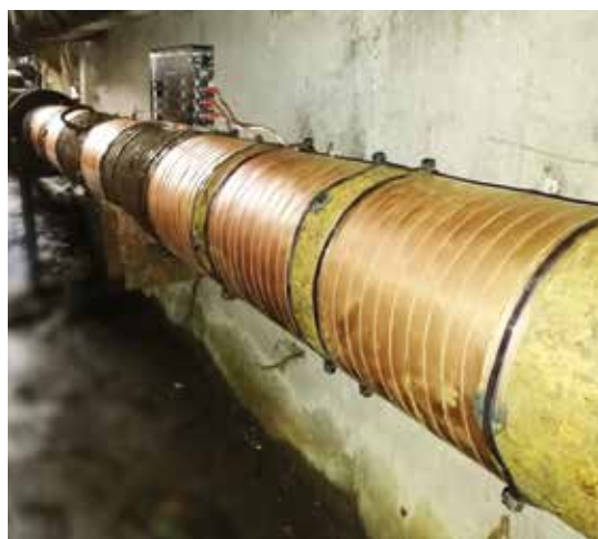
Vulcan S150安装在办公大楼及宿舍楼自来水主管道
