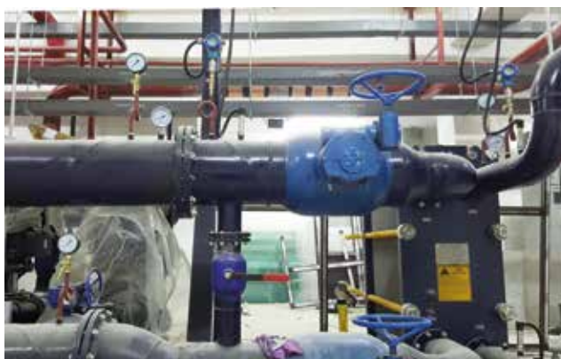
Vulcan S150安装在低区供热系统
