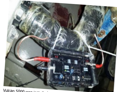
Vulcan 5000 was installed on the water inlet of the water recycling room.
