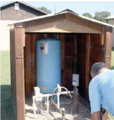
Home well water system
