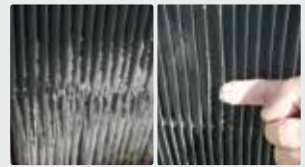
Cooling tower grids
