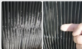
Cooling tower grids
