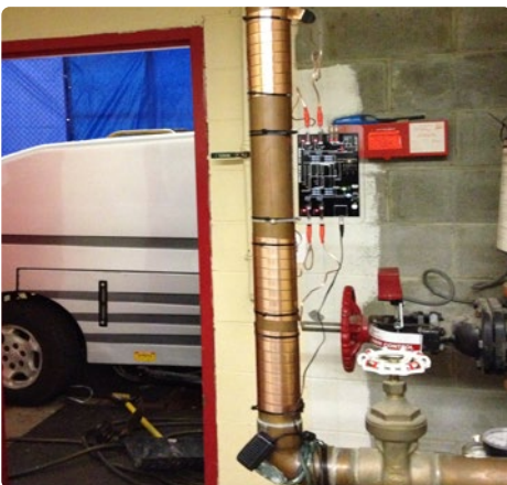
Vulcan S25 installed at Ice Land in New Jersey, USA.
