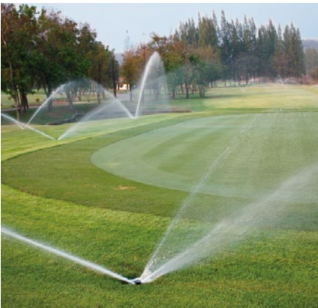
Sprinkler system on a golf course
