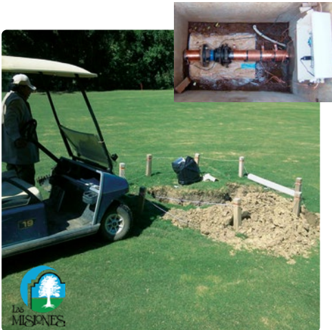
Vulcan installed underground at Las Misiones Golf Course
