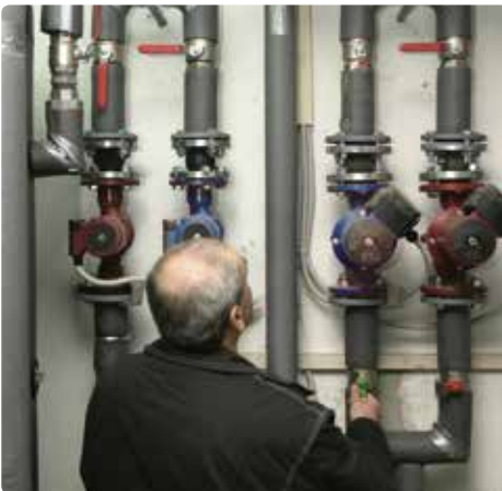
Piping system in an apartment building
