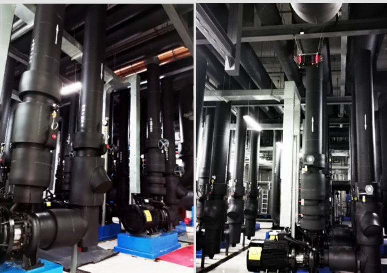
Vulcan S500 in Building A
