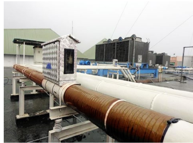
Vulcan S500 was located inside aluminum box and installed on a cooling tower main pipe in Supermal Karawaci.
