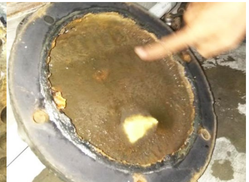
Inside of heat exchanger. Condenser end plate had lost all scale that was there previously. (Light spot at bottom is reflected light.)
