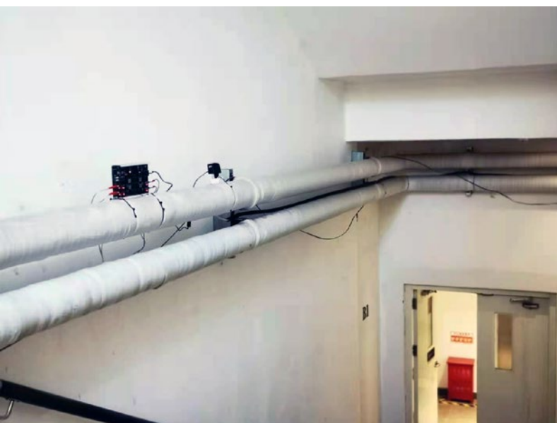
Vulcan S25 was installed on the main pipe leading to the heat pump in the stairwell.
