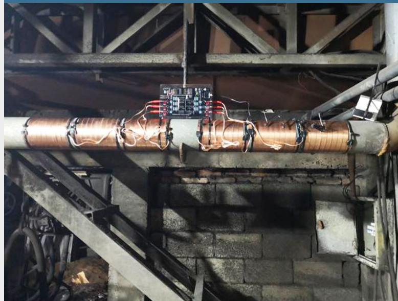
Vulcan S100 installed in the East Plant
