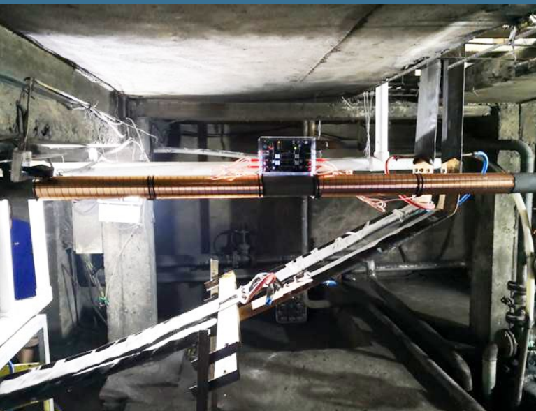
Vulcan S50 installed in the West Plant
