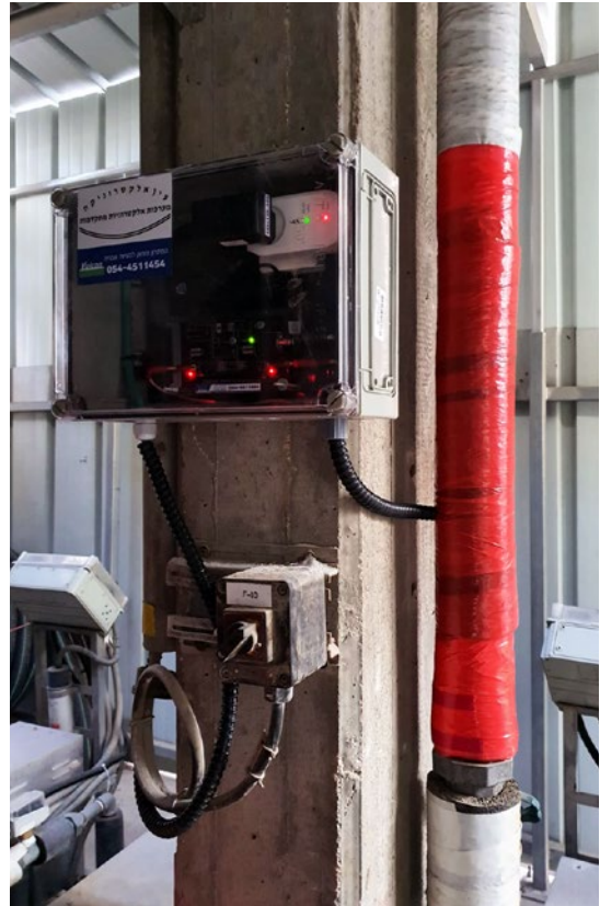
Vulcan 5000 was installed on the return water pipe of the heating system.
