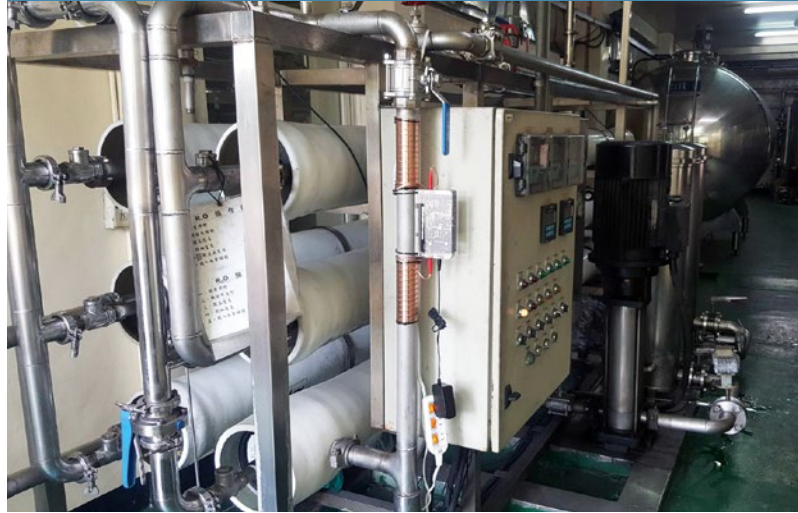
Vulcan 5000 installed for the RO reverse osmosis equipment to extend membrane life
