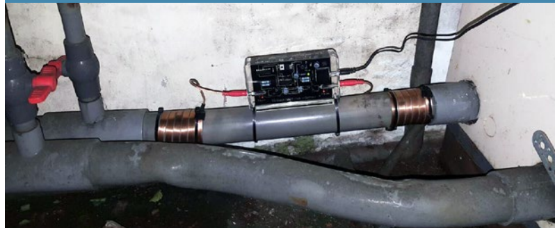
Vulcan 5000 installed on the 2" circulating water pipe
