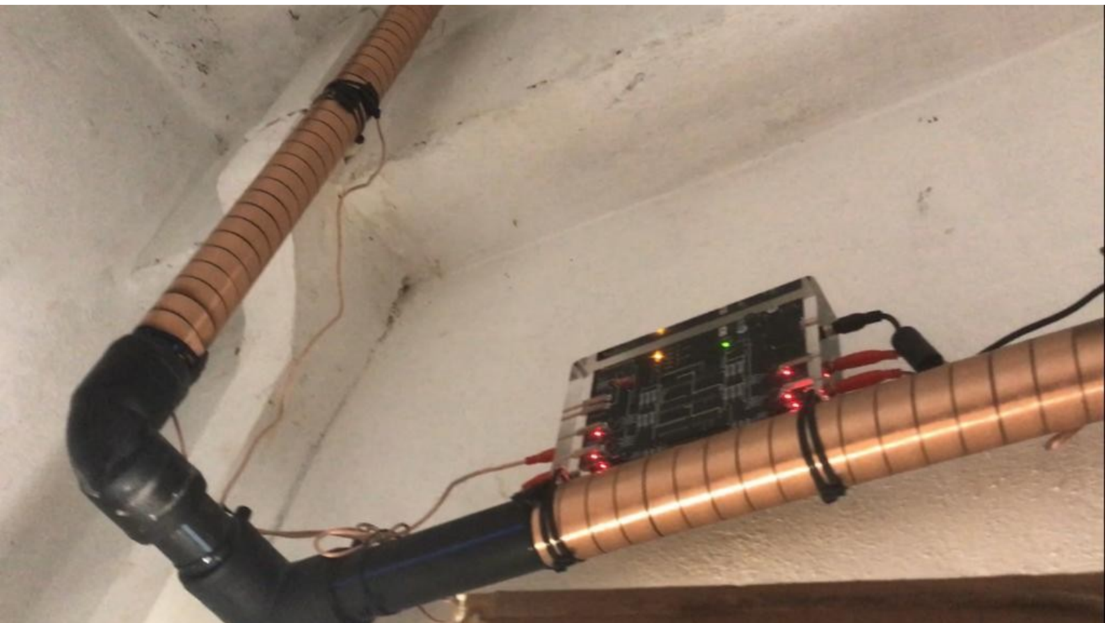
Vulcan S25 at cold water main pipe
